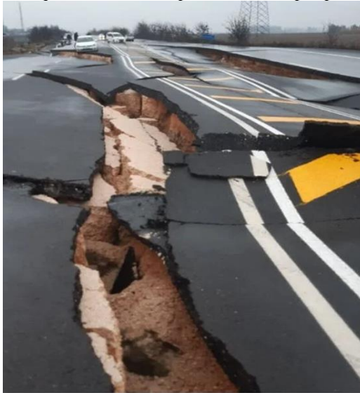
Figure 1. Cracks on Hatay-Reyhanlı highway due to Kahramanmaras earthquakes
